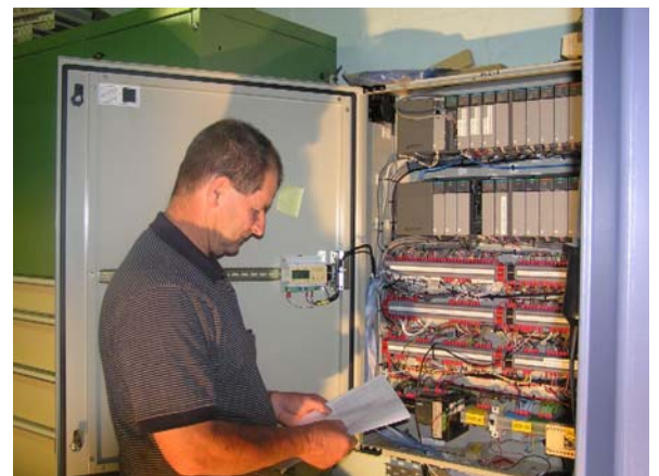
Figure 8: Ray Kimlin and PLC3, which controls cooling and the machine sequencer.
